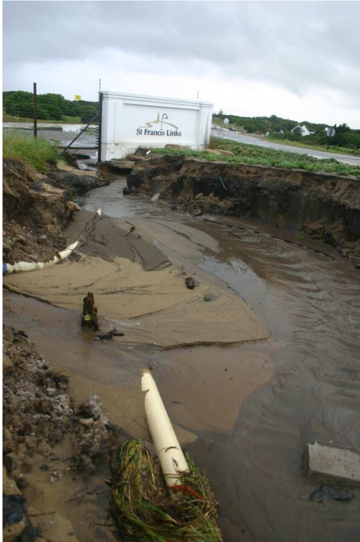
Figure 3. Damage to infrastructure associated with the transport of sand and water from the Easter Valley Bottom wetland after the high rainfall event in November 2007.
