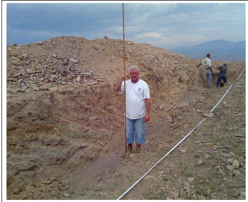
Figure 4 : Trenching conditions in Bokkeveld shales. Onset of heavy ripping conditions for rock excavation at approximately 1.5m.
