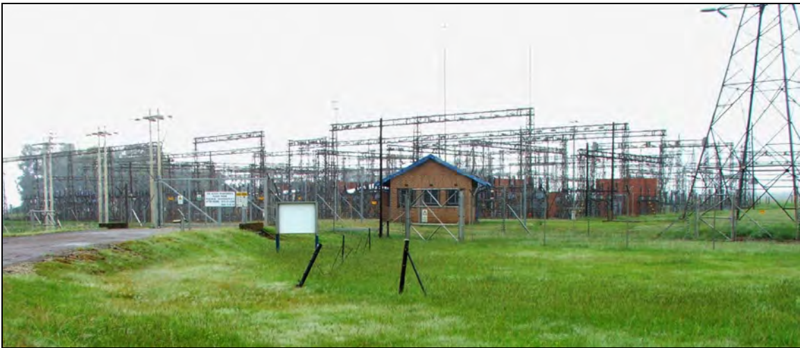
Figure 3: Existing Westgate Substation
