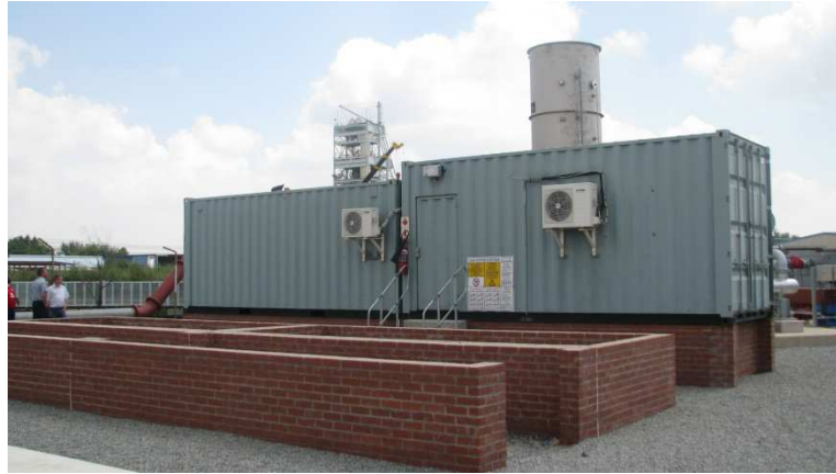
Figure 10: Existing Shaft 1: Generators, Flare & water cooling systems
